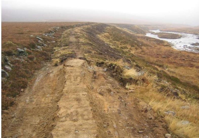
Glen Dee, former vehicle track after and during restoration back to footpath width. Photo credit: National Trust for Scotland
